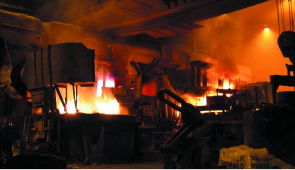
Fig. 4: Steel mill with two electric arc furnaces; each furnace consists of a refractory lined hearth, in which the feedstock is molten down using one or more graphite electrodes which enter the furnace through the refractory-lined roof; http://en.wikipedia.org/wiki/Electric_arc_furnace EAFs are the heart of a special steel production. To follow charge formation and meltdown is very spectacular but dangerous; melt capacity is commonly between 50 to 80 t, but can go up to 300 t. Tungsten is added to the furnace charge either as tungsten scrap or in the form of ferrotungsten
