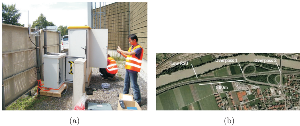
Figure 4.20: (a) Mounting of the antenna and (b) satellite photo of the low RSU
