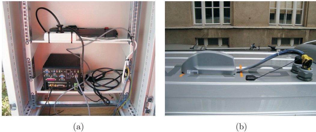
Figure 4.15: (a) RSU installation and (b) OBU antenna
