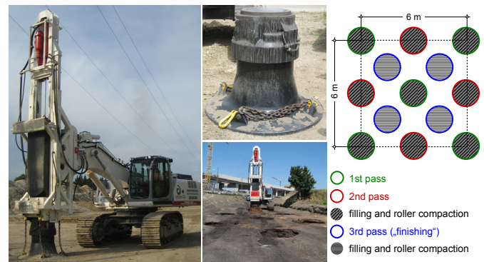
Figure 1. Rapid Impact Compactor (left), impact foot with driving cap (center top), points of compaction (center bottom), and compaction process (right).
