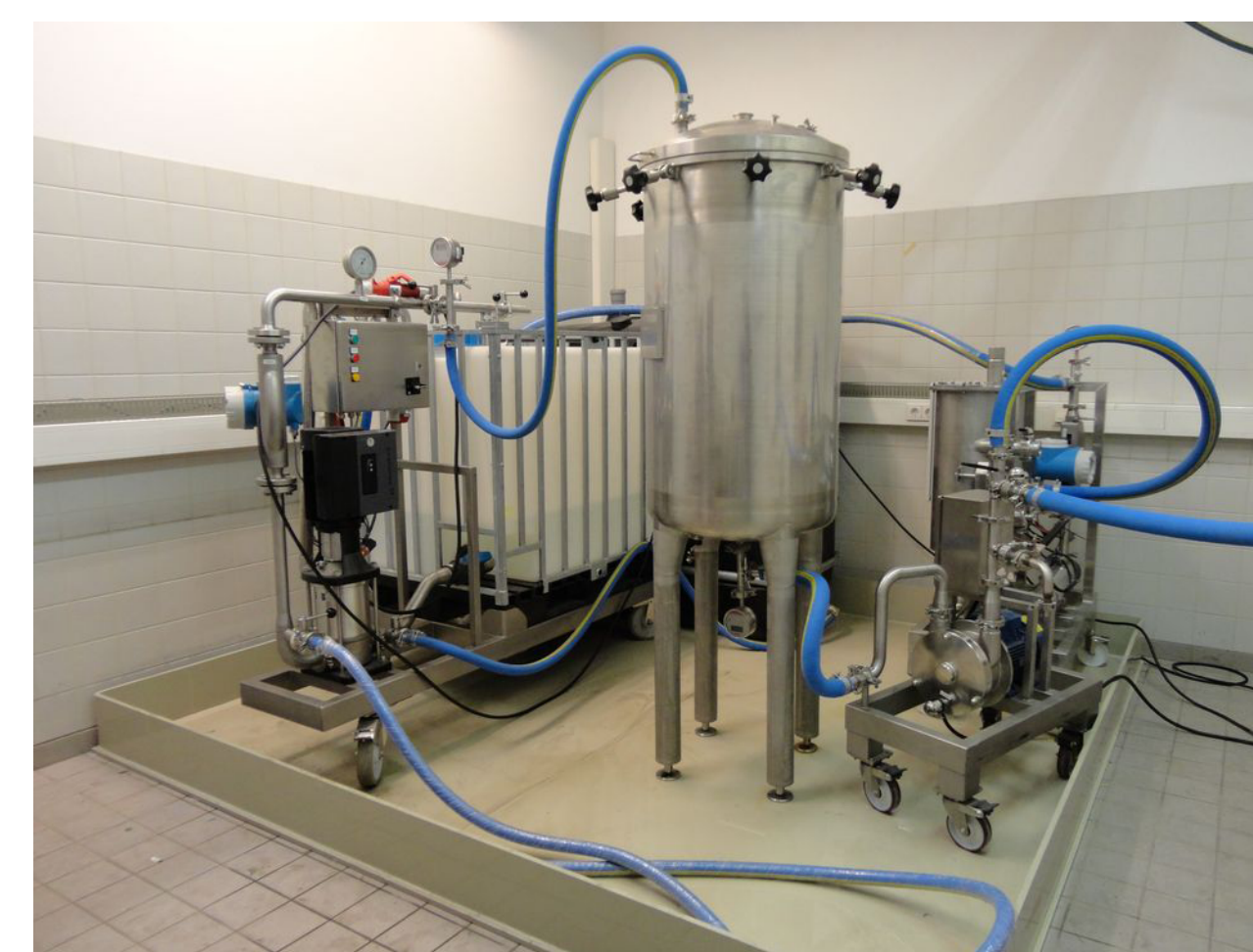
Fig. 4: Assembled PATOV testing facility
