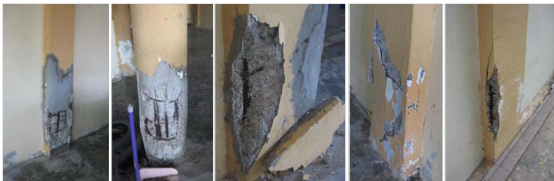
Figure 1. The concrete damage and reinforcing damaged by corrosion of column.
