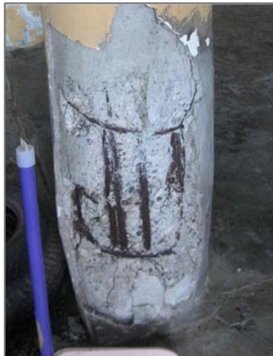
Figure 2. Reinforcing ties are broken due to corrosion.
