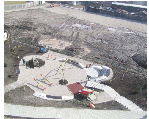
AFTER: Educational areas with playground with sports field under leveling works. Photograph taken from top floor of a newly constructed social housing unit.
