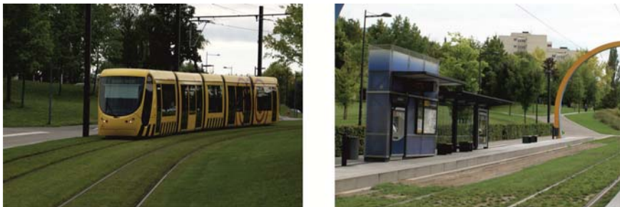
Figure 5. Perfect green track (left) in Mulhouse and the damaged green track at a terminal stop (right) caused by (too) long idle time and multiple mechanical impacts by trespassing passengers.
