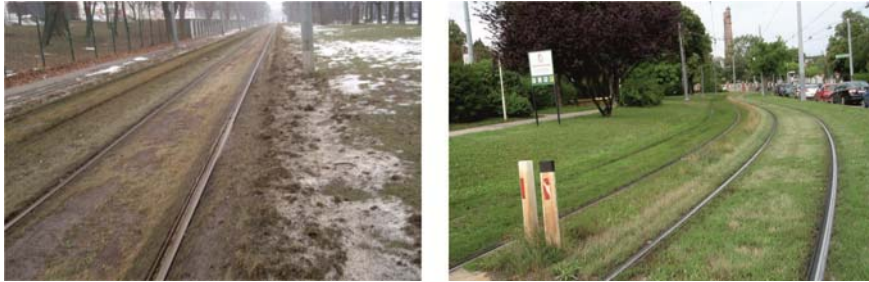
Figure 6. Damages by winter service: Grass sods peeled from the track and dumped alongside the track (left). View of the test field at Lainz before re-cultivation (right).
