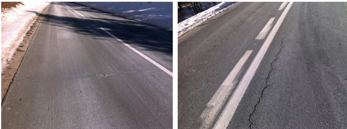
Fig. 1. Babno Polje, February 2012: (a) Transversal thermal crack, (b) Longitudinal crack at the wheel tracks.
