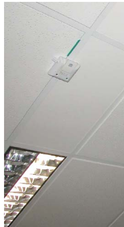
Figure 15: Occupancy/light status logger
