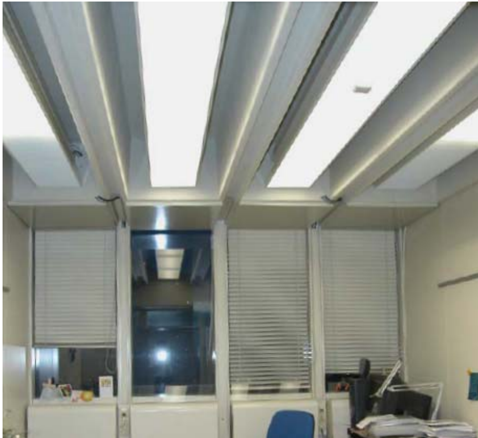
Figure 10: An office room in VIC with 12 fluorescent fixtures and 4 blinds
