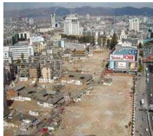
Pic. 4: Construction and development in the centre of Kunming city, Yunnan Province. Large areas of bare, uncovered soil are exposed for many months.
