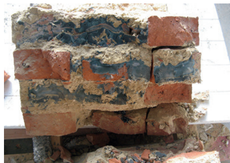
Abb. 6: Verfüllung von Mikrozement in den Spaltflächen des geprüften Bohrkerns; Fig. 6: Areas of microcement between the bricks visibly after the compression test
