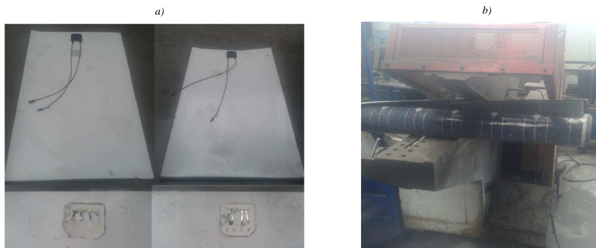
Fig. 10. a) Removed aluminium frames and junction boxes, b) PV modules cutting into two halves.
