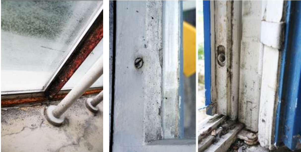
Figure 06 and 07. Source: P.GOOD Architects, Vienna. Several damages at the Rietveld houses
